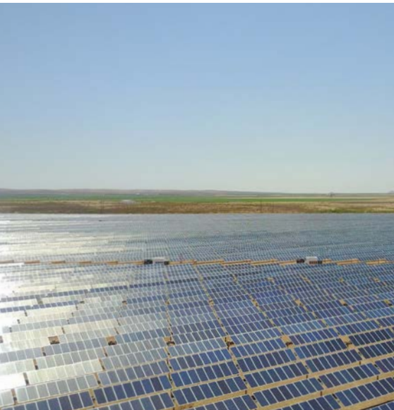
Los Santos Solar I, a solar park in northern Mexico, avoids around 16,500 tonnes of carbon emissions per year.
